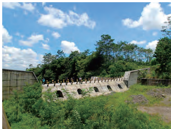
GED1 Check Dam
